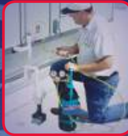
Clean condensate drain lines with the Sludge Blaster®
