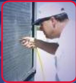
Blow off coils with Sludge Sucker® Blowgun
